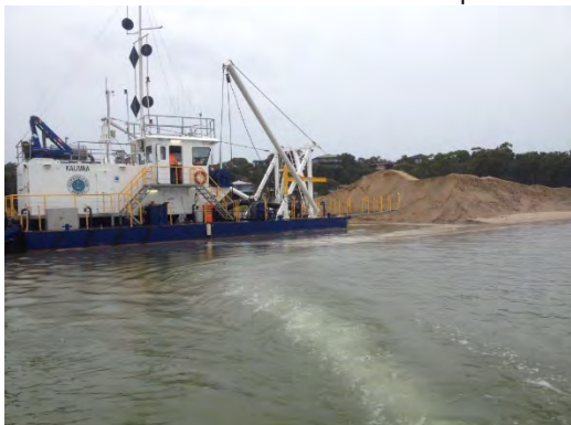
g) CSD Kalimna dredging Seagull Drive boat ramp access at Loch Sport for DELWP.
