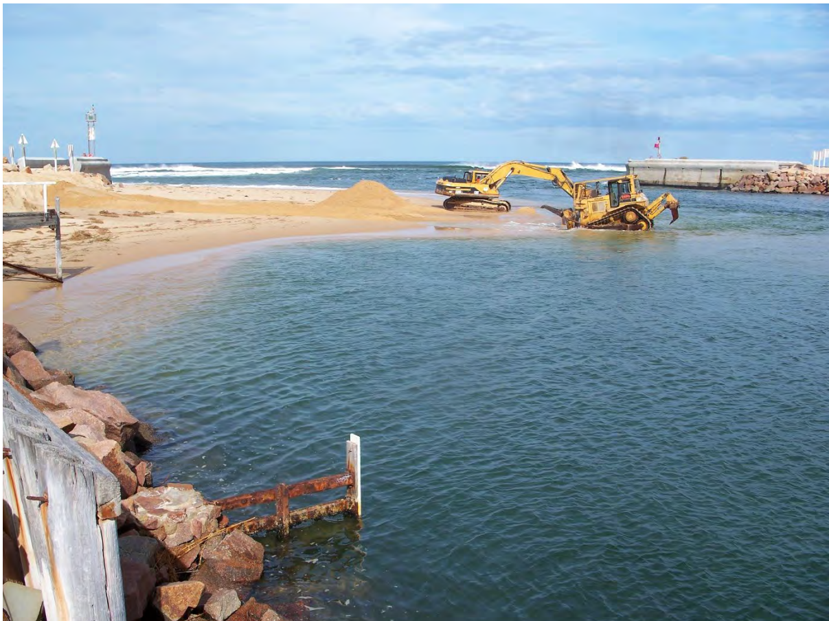
Figure 3: Entrance Channel severe sand accumulation in May 2007 (Lakes Entrance)
