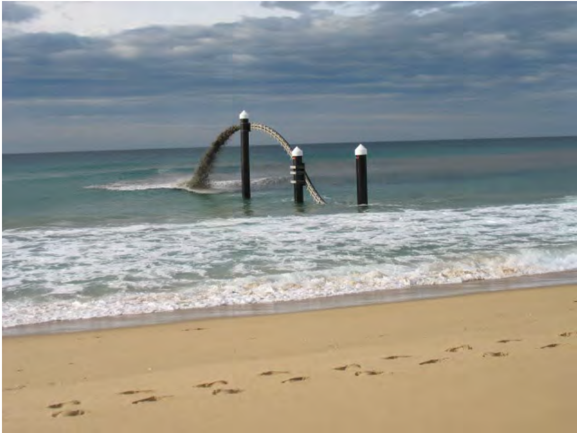
Figure 53: Eastern outfall (discharge location)
