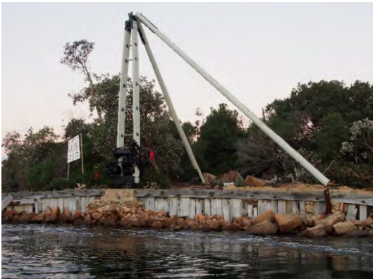
e) Heritage 'Jib' Crane restored by Parks Victoria with assistance from Gippsland Ports including sand nourishment of site for erosion protection.
